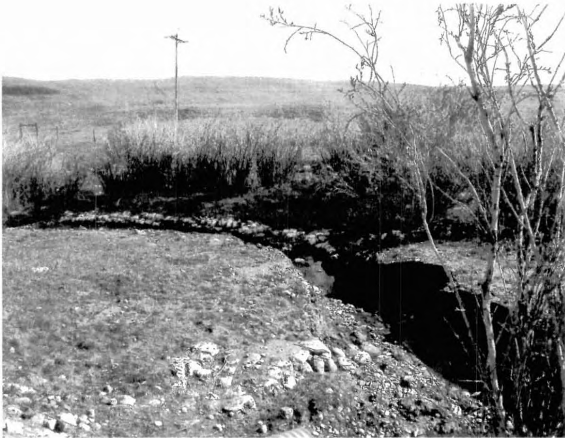
View to the east showing remediation area just east of the culvert. Note that vegetation is filling in on the north bank after the excavation and bank reconstruction.
