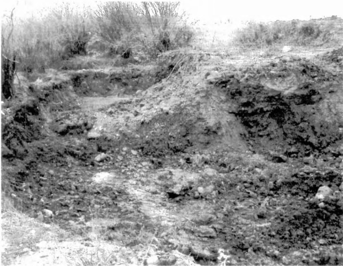
View of the southwest walls of the excavation during remediation activities. Note the crude-impaired zone of soils. All visible remnants of crude were removed from the west side of the stream's banks and bed to a depth of approximately 8 feet.
