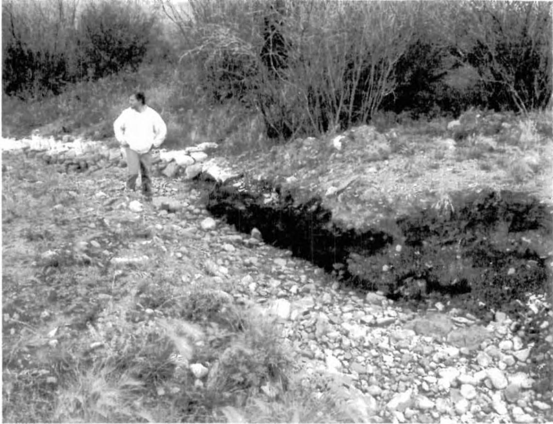
View to the east showing the bank and the pre-vegetation state following bank reconstruction. Sandbags on the east bank of the stream were placed in March 2005. Residual crude deposition was noted to have occurred between the time of the bank reconstruction and the September 2005 field review.
