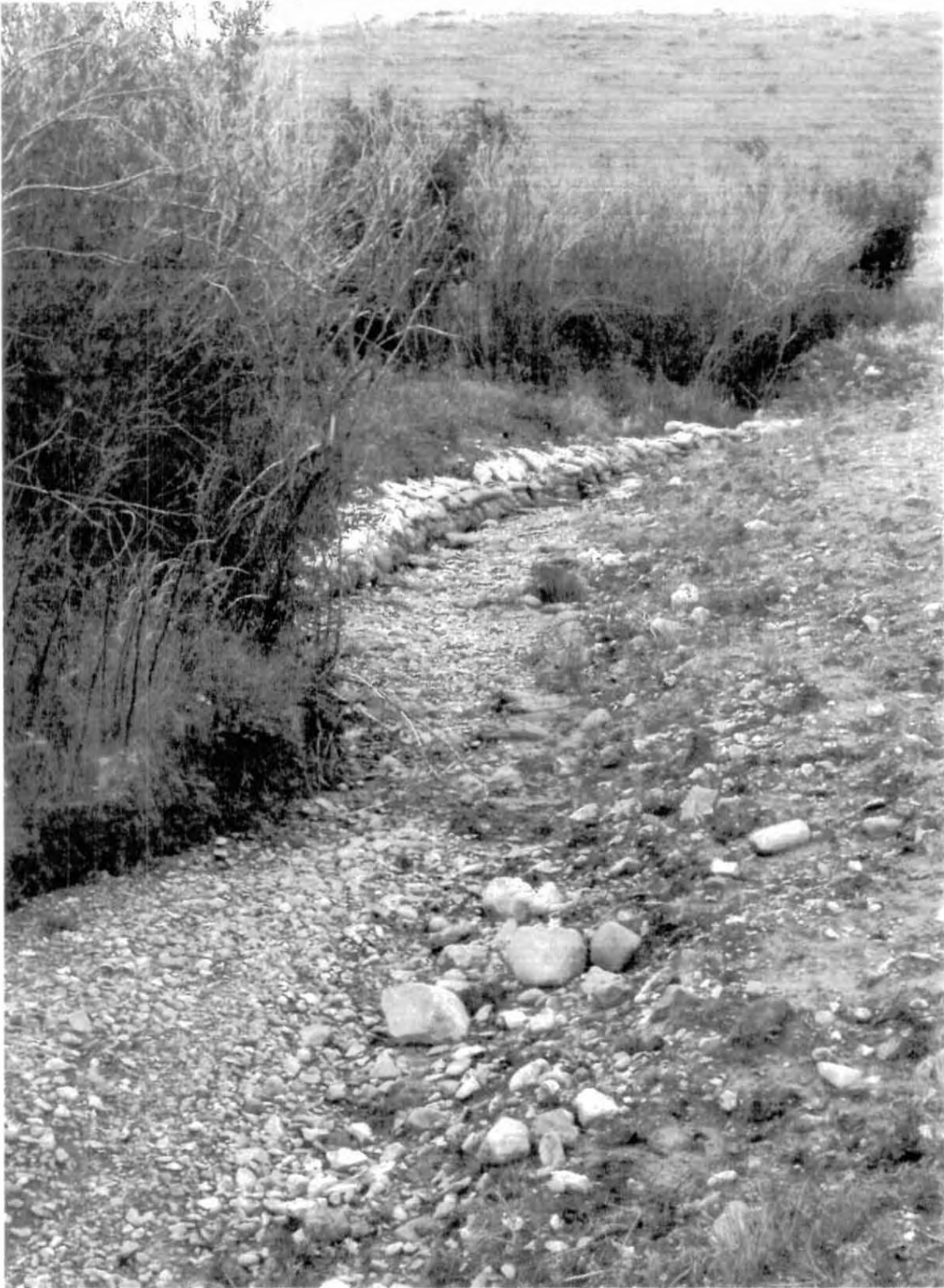
View to the south showing the stream channel following stream and bank reconstruction. Sandbags on the east bank of the stream were placed in March 2005. Photo taken: September 29, 2005
