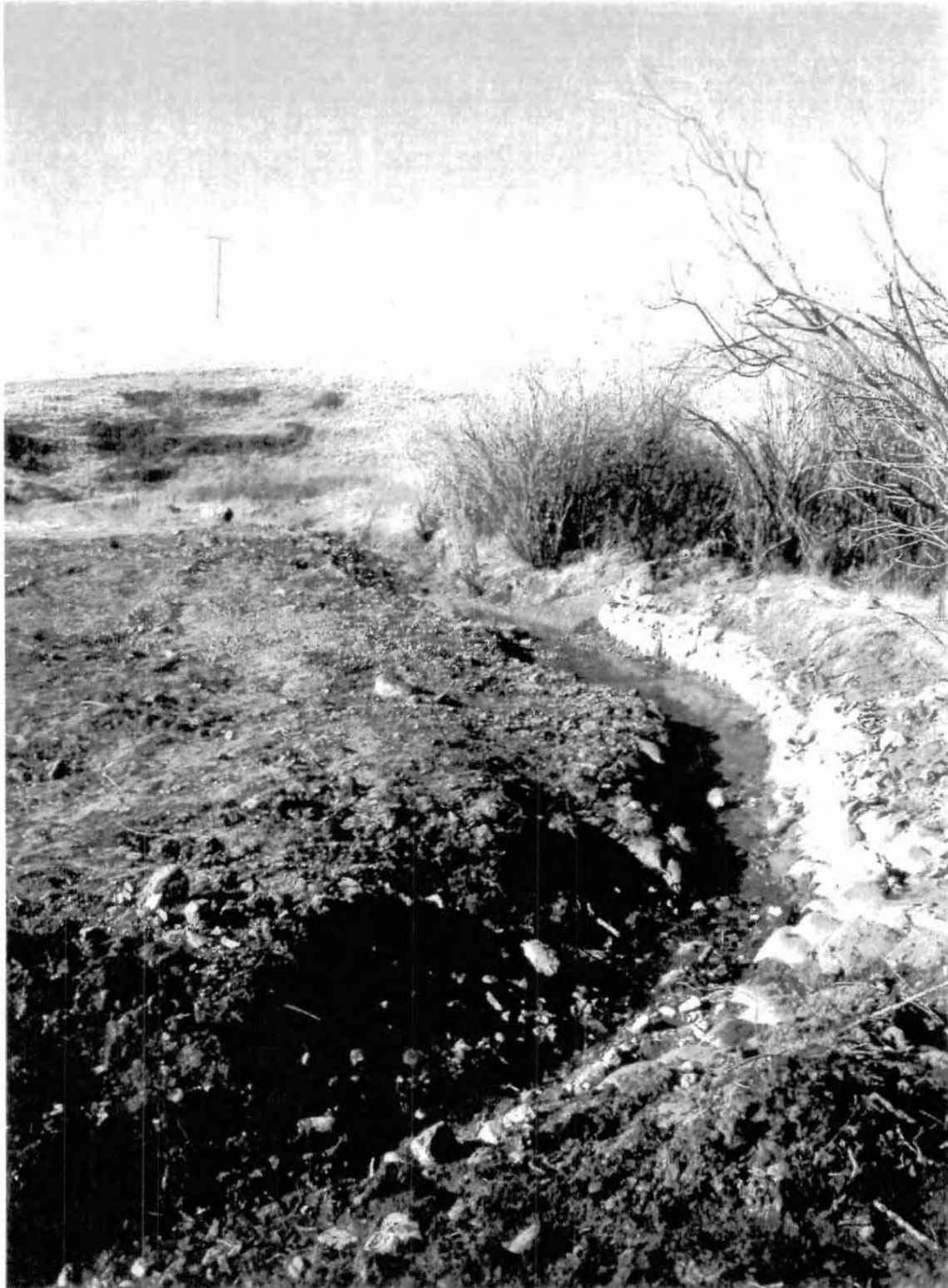
View to the north showing the pre-vegetation state following bank reconstruction. Sandbags on the east bank of the stream were placed in March 2005.
