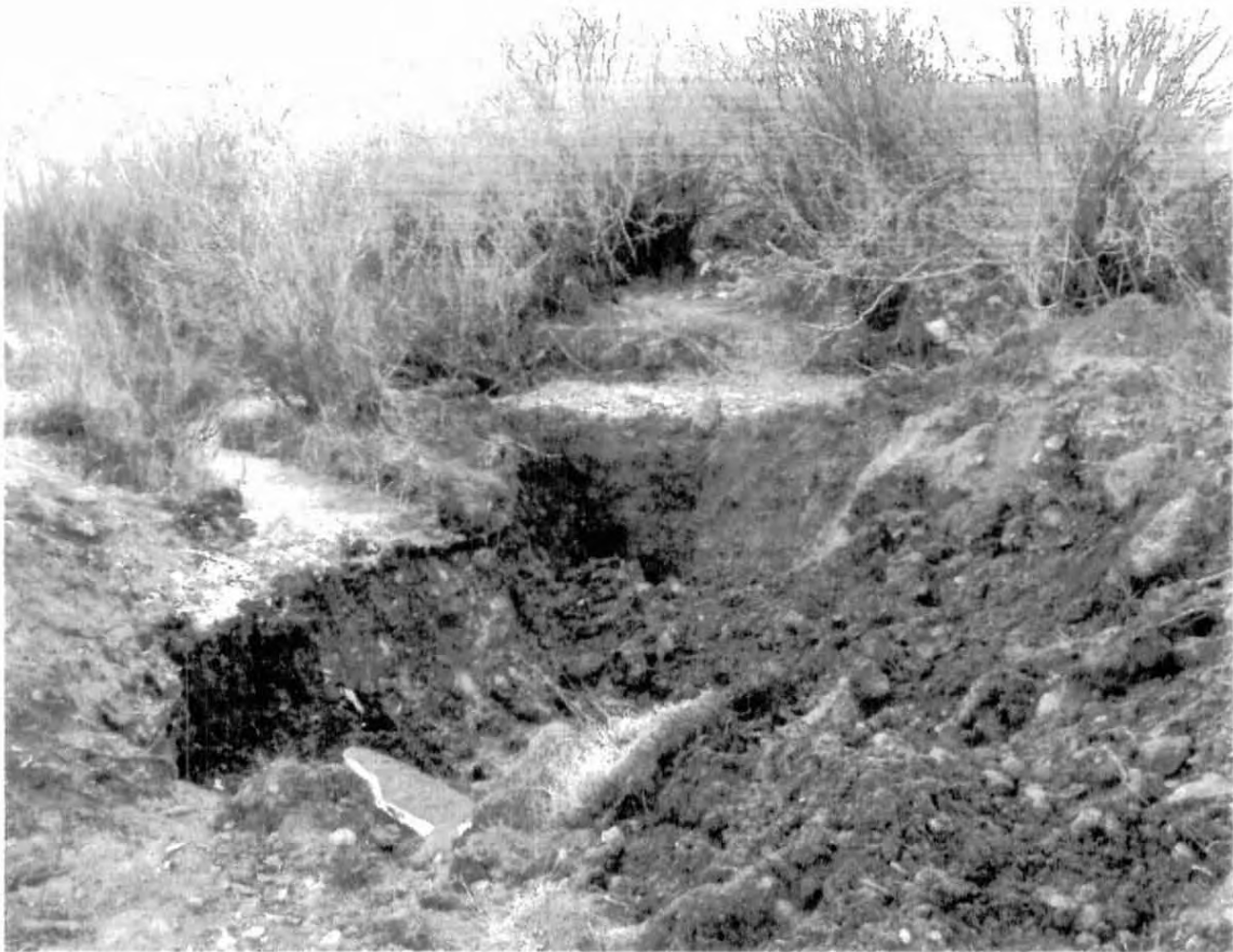
View of the south end of the excavation during remediation activities. Note the crude-impaired zone of soils. The crude material generally reached a depth of approximately 6 to 7 feet. Photo taken: December 10, 2004
