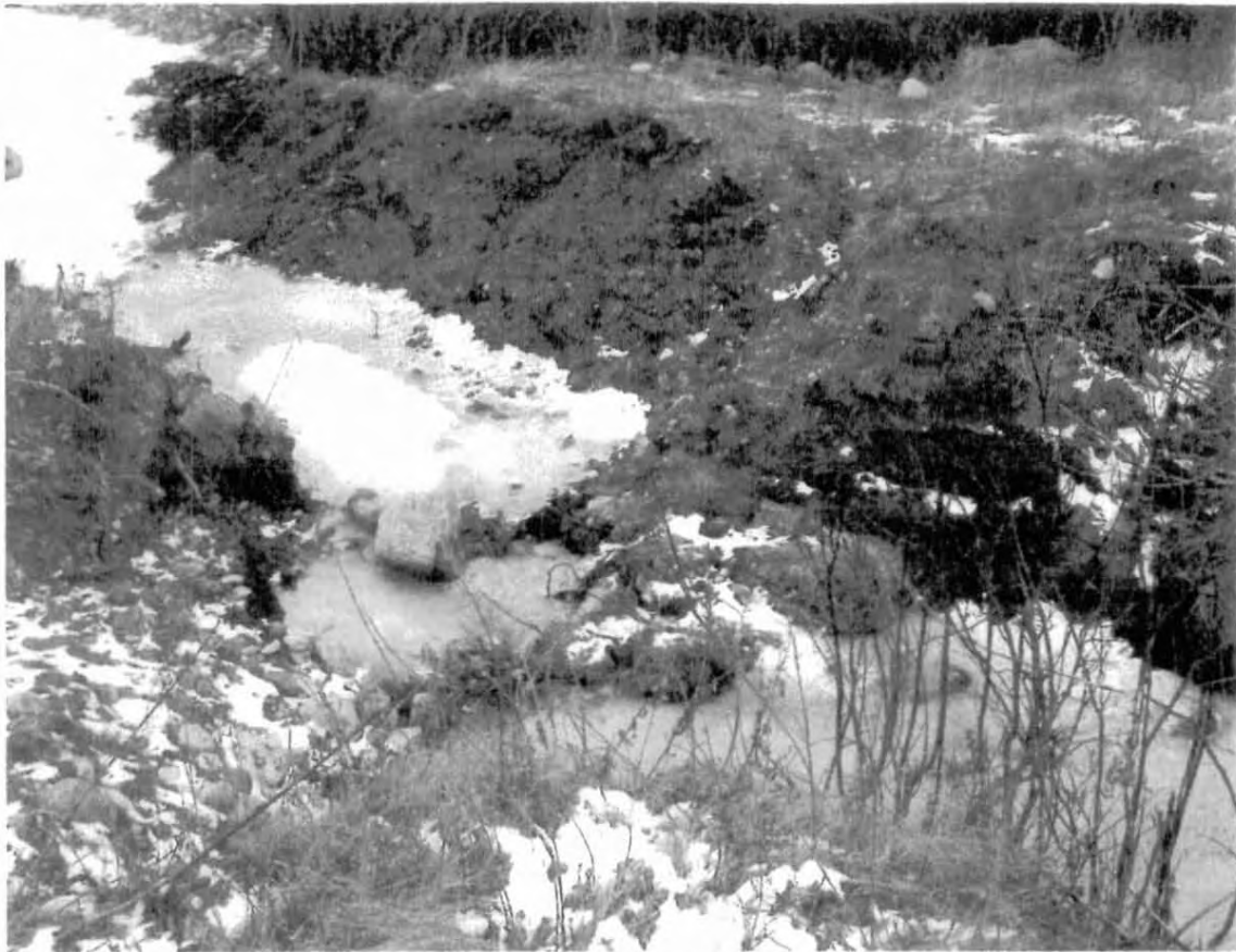
View to the southeast of the stream bed and banks, pre-excavation. The disturbed area of the banks is where the fiberglass pipeline was excavated and capped on either end to prevent any additional release from residual crude in the lines.
