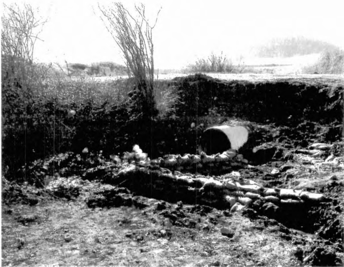
View to the west showing the pre-vegetation state following bank reconstruction. Sandbags on the northwest bank of the stream were placed in March 2005. Photo taken: March 15, 2005
