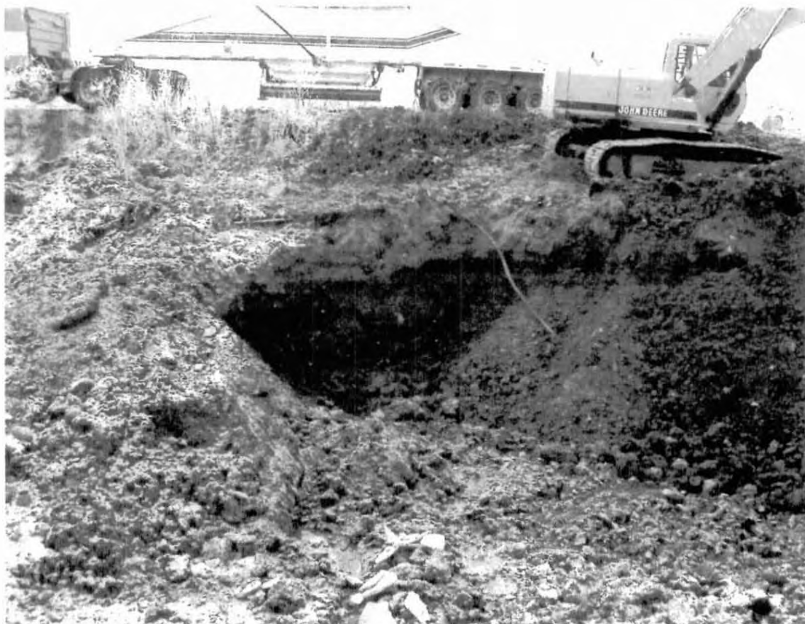
View of the west wall of the excavation during remediation activities. Note the crude-impaired zone of soils. All visible remnants of crude were removed from the west side of the stream's banks and bed to a depth of approximately 8 feet.
