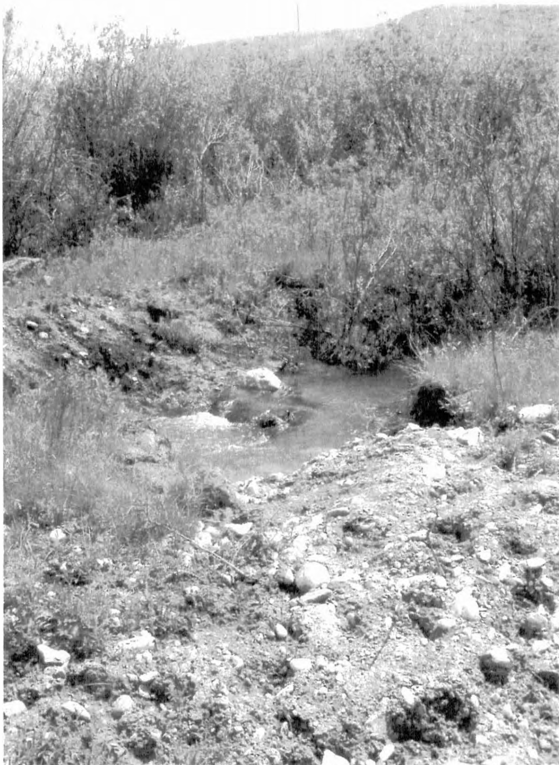
View to the south of the flowing stream at the approximate southern end of the planned excavation area. The ground disturbance (center left) was caused by the excavation of the fiberglass pipe in order to seal off the ends to prevent further release.
