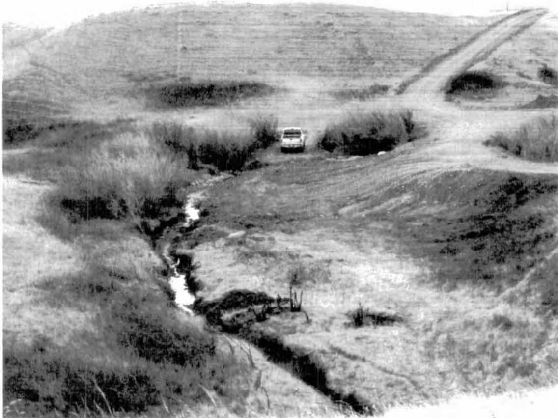
View to the south showing the pre-vegetation state following bank reconstruction. Sandbags on the east bank of the stream were placed in March 2005. Photo taken: March 15, 2005
