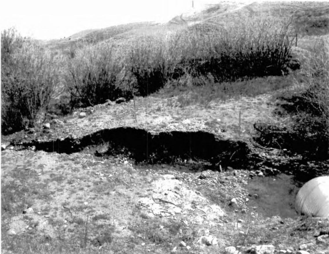
View to the southeast showing remediated area just below culvert. Note that vegetation on both banks (north and south) is beginning to fill in where topsoils were replaced after the excavation and bank reconstruction. Also note the stream cuts beginning to develop.
