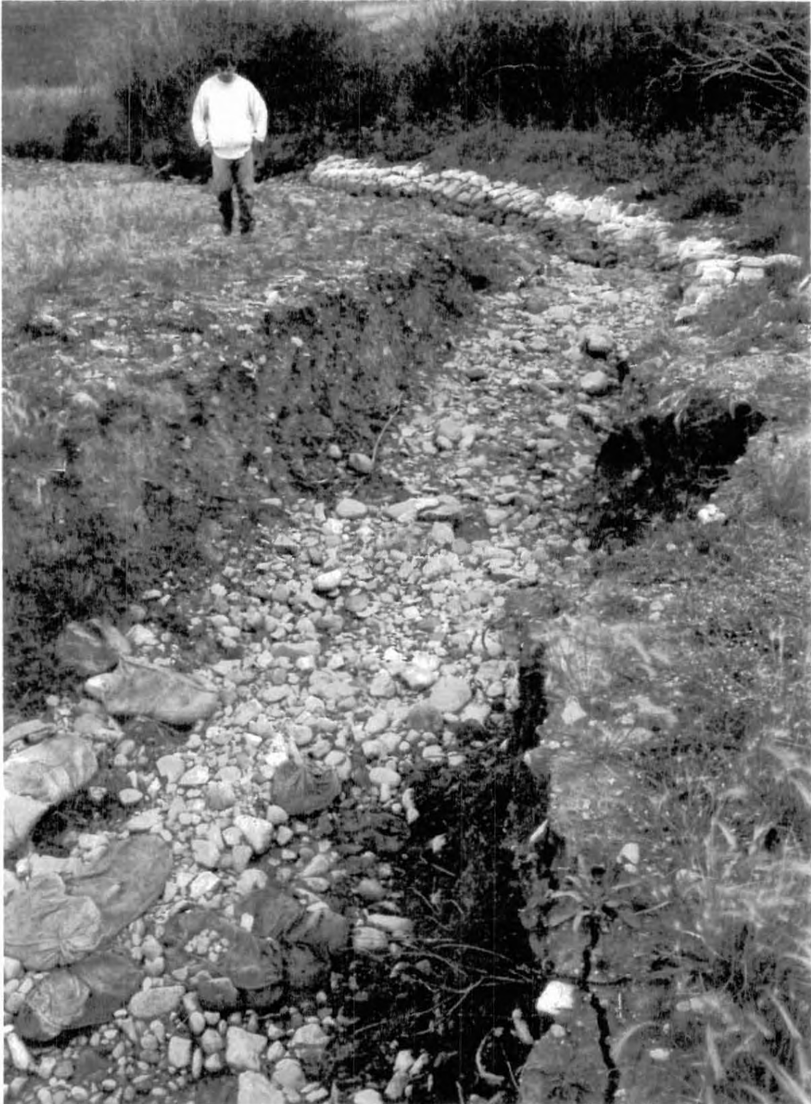
View to the northeast showing the bank and the pre-vegetation state following bank reconstruction. Sandbags on the east bank of the stream were placed in March 2005. Photo taken: September 29, 2005
